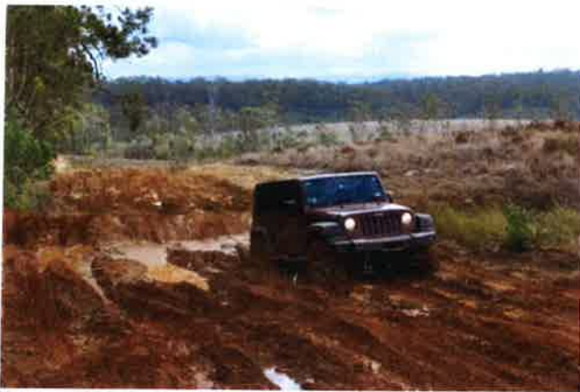
Figure 1 Severe erosion and runoff
