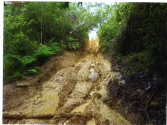
Figure 2 Severe erosion and runoff on fire trail
